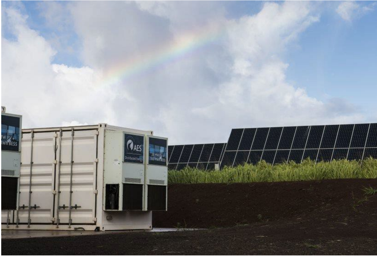
Figure 14. A Solar PV System Paired with Battery Storage
