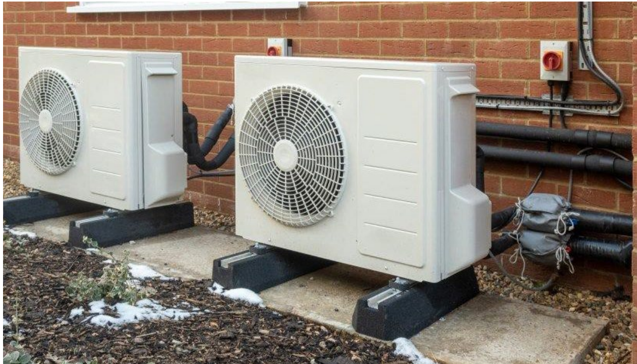
Figure 10. Air Source Heat Pumps
